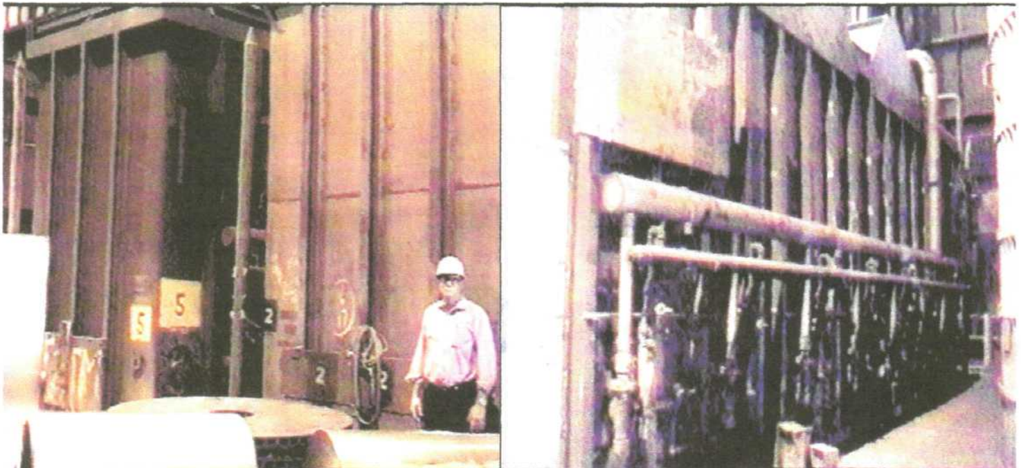
Burners on right side of #5 Furnace
