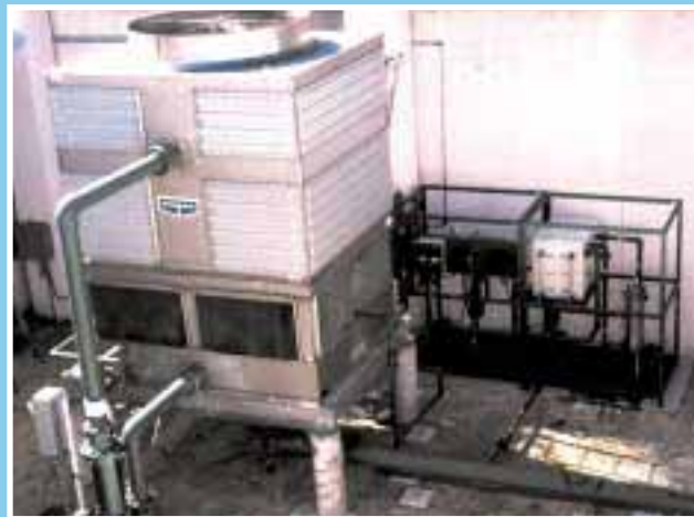
RT-1000-K, ACV-6-K, & CT-400-ZB Environmentalist/Zero-Bleed® on a Comfort Air Cooling Tower
